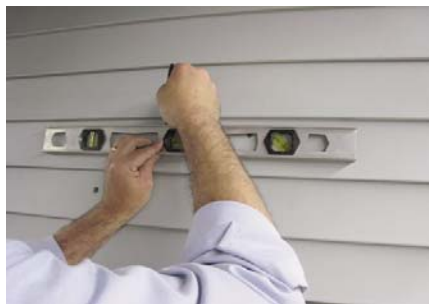
DRILL (4) 1/2" CORNER HOLES THROUGH WALL FROM INTERIOR AND CONNECT HOLES ON EXTERIOR WITH A LEVEL.
